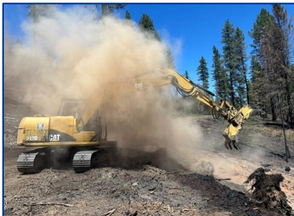
Machinery pulling apart the ash pit that the Engine Boss had stepped into three weeks after this injury incident occurred. Note the steam cloud rising from the ash pit, illustrating how hot it still was.
